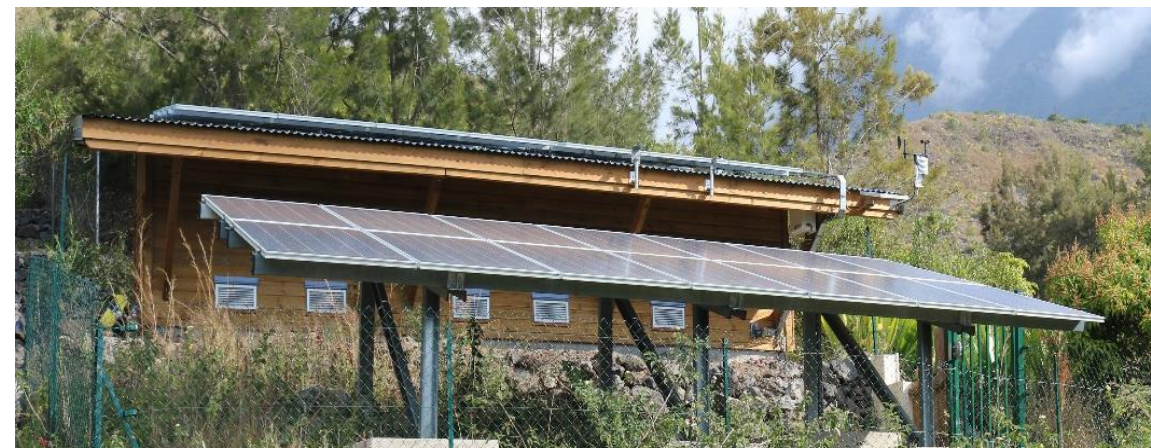
Figure 9 – Microgrid solar plant
